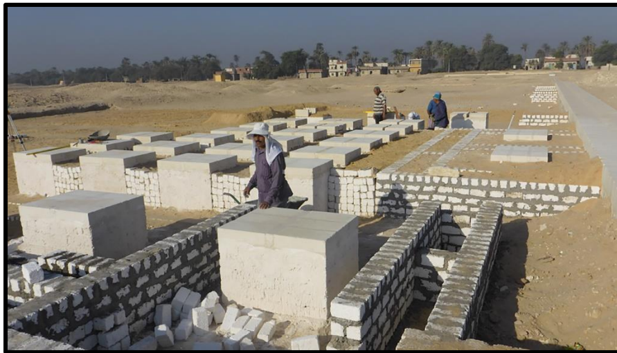
Figure 5: Nearing the end of the autumn 2022 season, view to the west. The walls of un-mortared small blocks between offering-tables are a temporary measure to hold back the sand fill that recreates the original floor level.
