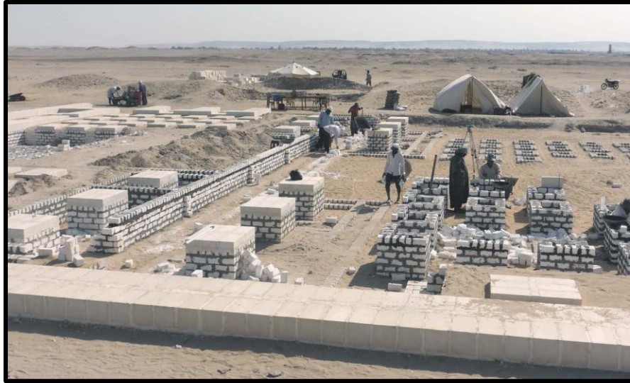
Figure 4: Mid-season, autumn 2022. The builders work over an area of the temple foundations previously cleaned and recorded. First come the new foundations built from small local limestone blocks. Then a final layer of Tura-limestone blocks. Finally the ground level is built up using sand spread between the walls. View to the south.
