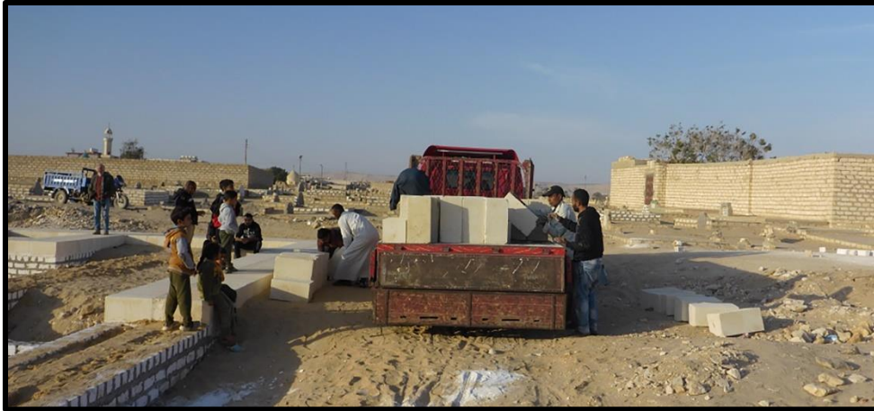
Figure 2: A lorry delivers blocks of limestone from the Tura quarries to the rear of the temple. View to the north.
